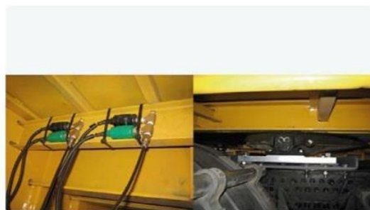
Figure 23 Air Pressure (left) and Load Cell axle load OBW sensor (right)
