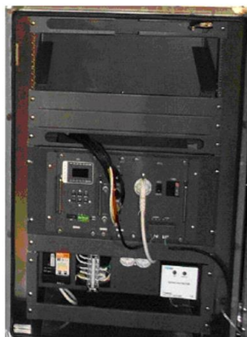
Controller case: Controller, Surge Protector, Communications Equipment
