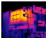
Thermograph of Component
